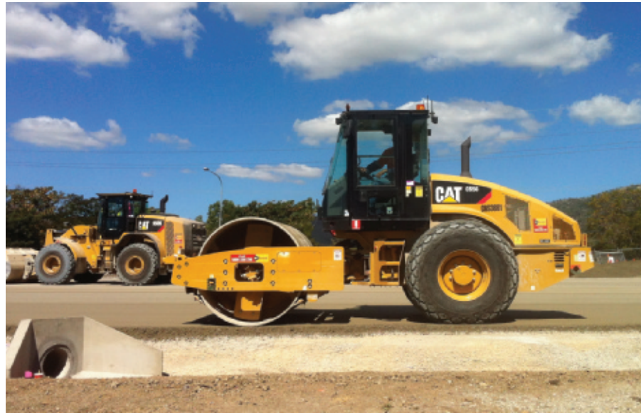
FIGURE 1.2 Soil compaction for a highway construction project (Courtesy of N. Sivakugan, James Cook University, Australia)
